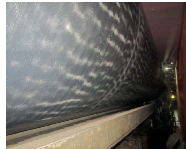
Figure 1: Chatter marks on a dryer cylinder caused by uneven grinding
