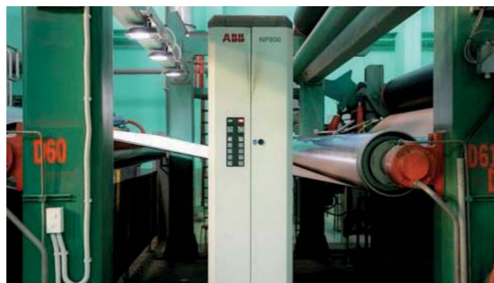
An ABB Network Platform 800 scanner is also installed to improve production quality and reduce downtime
