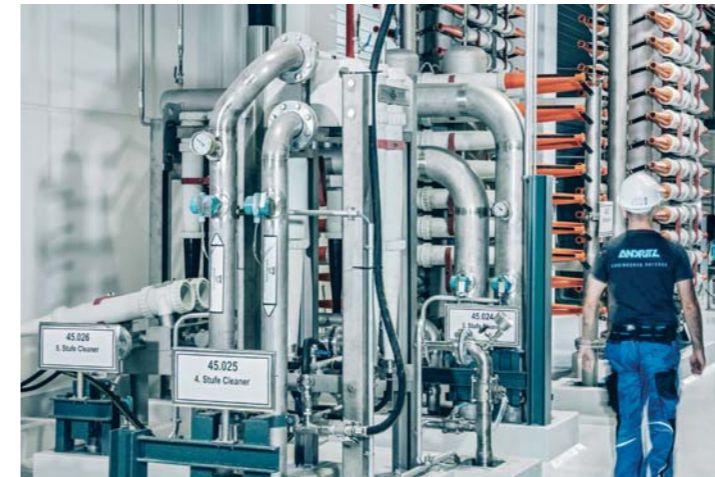
Five-stage cleaner system for the new PM3
