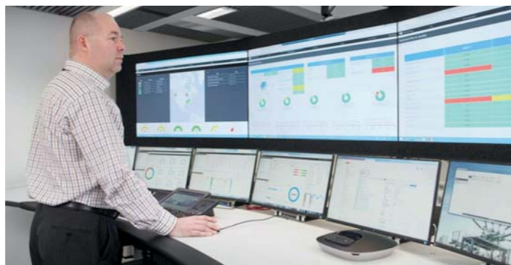
An operator at ABB's collaborative Operations Center in Helsinki, Finland
